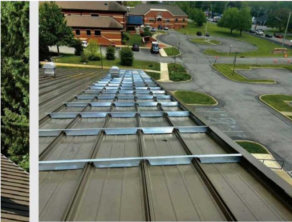
A new metal roof system was installed over the existing roof of the Fishkill Recreation building.
