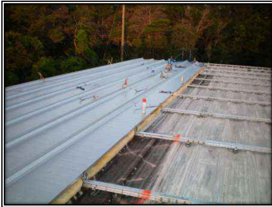
Photo N: New sub-purlins and insulation have been installed, which is then followed by the placement of the new roof panels.
