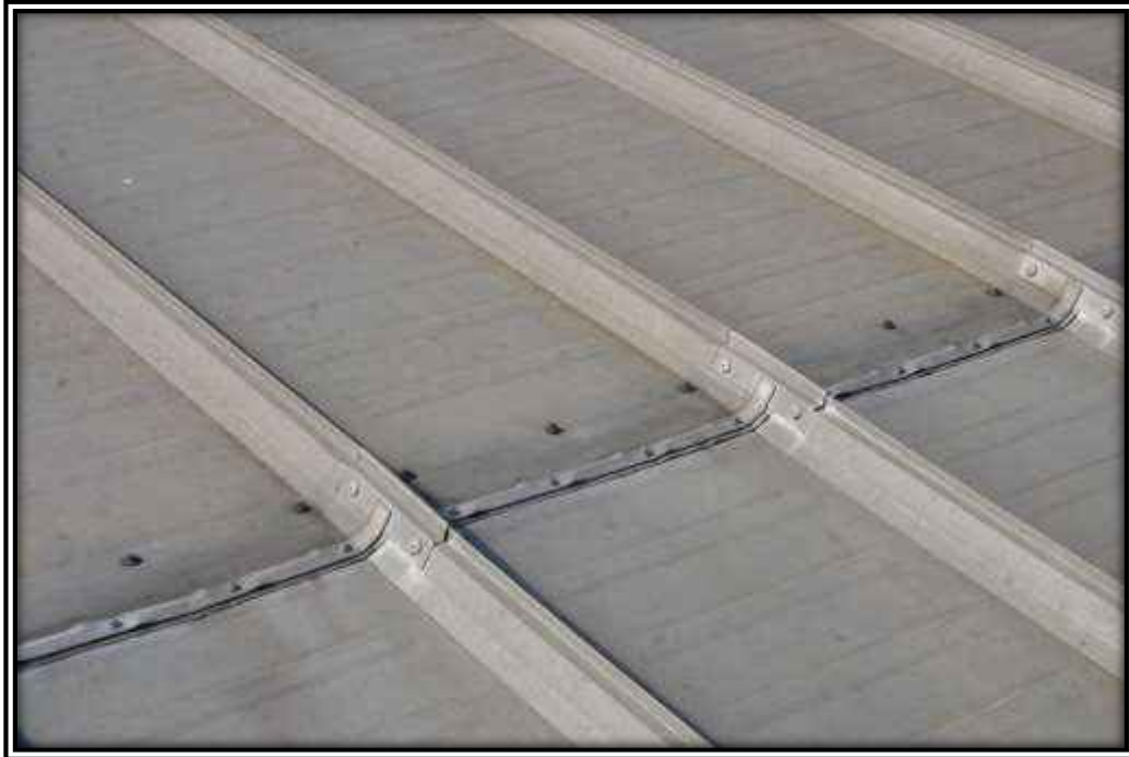
Photo B: This thirty year plus trapezoidal standing seam roof still performing.
