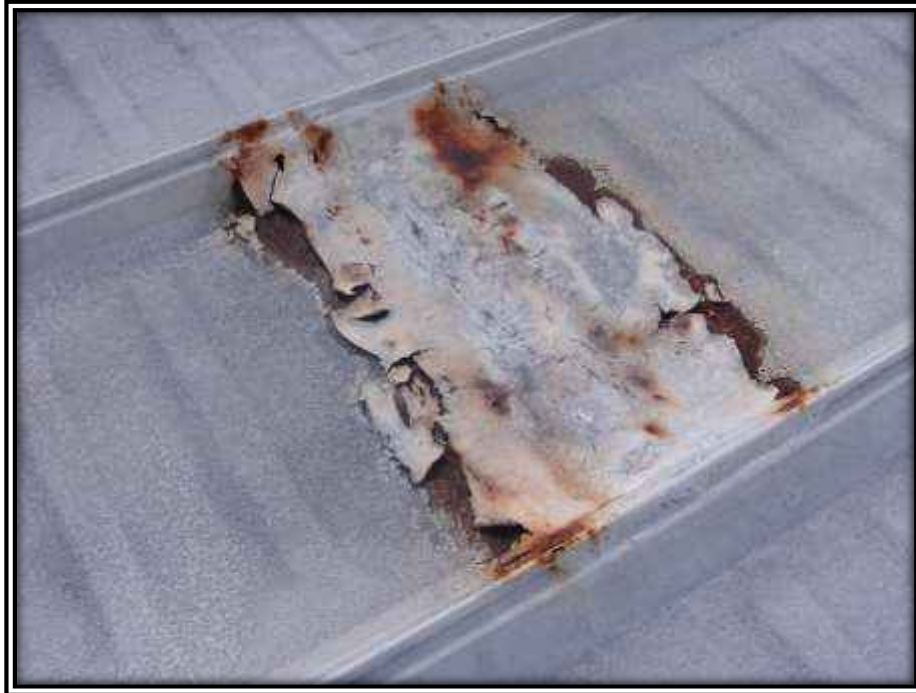
Photo H: Coating applied to the transverse lap seam, peeled and allowed moisture to enter under the coating, but not out. This resulted in the deterioration of metal roof panel.
