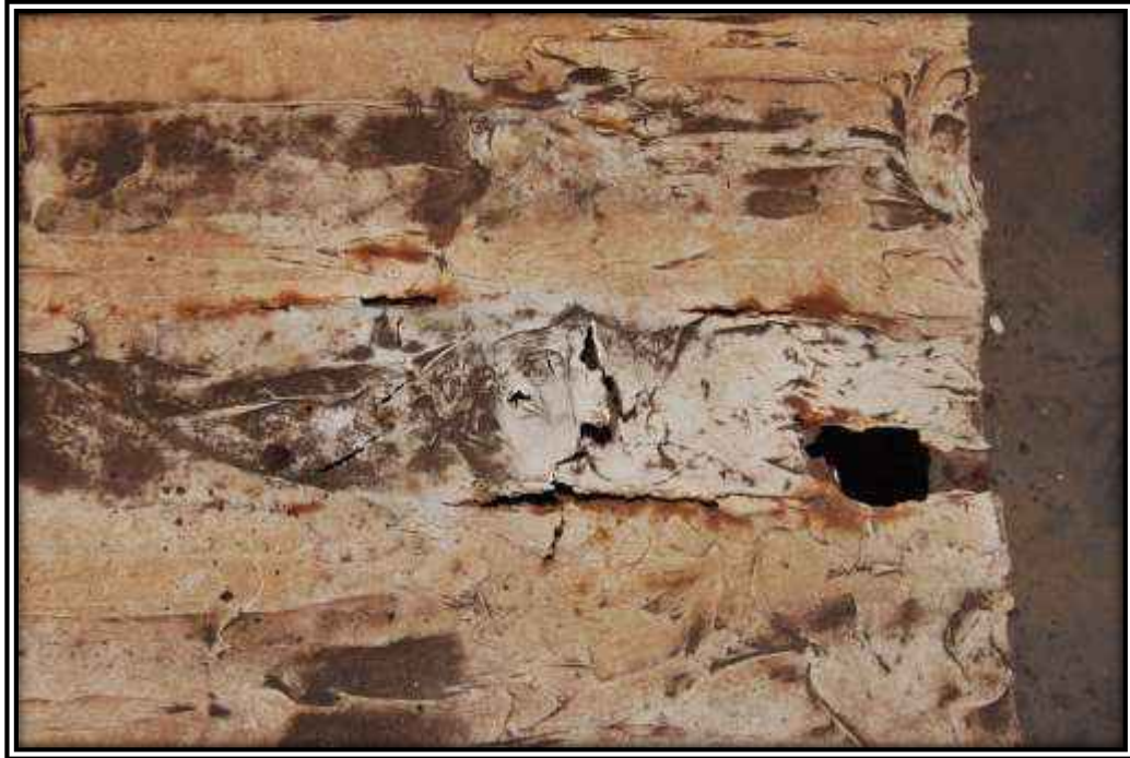
Photo G: The coating in this photo concealed a nearly rusted out panel that created a life-safety concern. The panel should have been repaired prior to coating.
