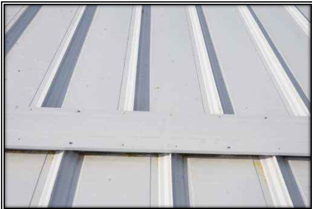
Photo C: This trapezoidal seam roof panel, with a pre-finished coating is a recent installation.
