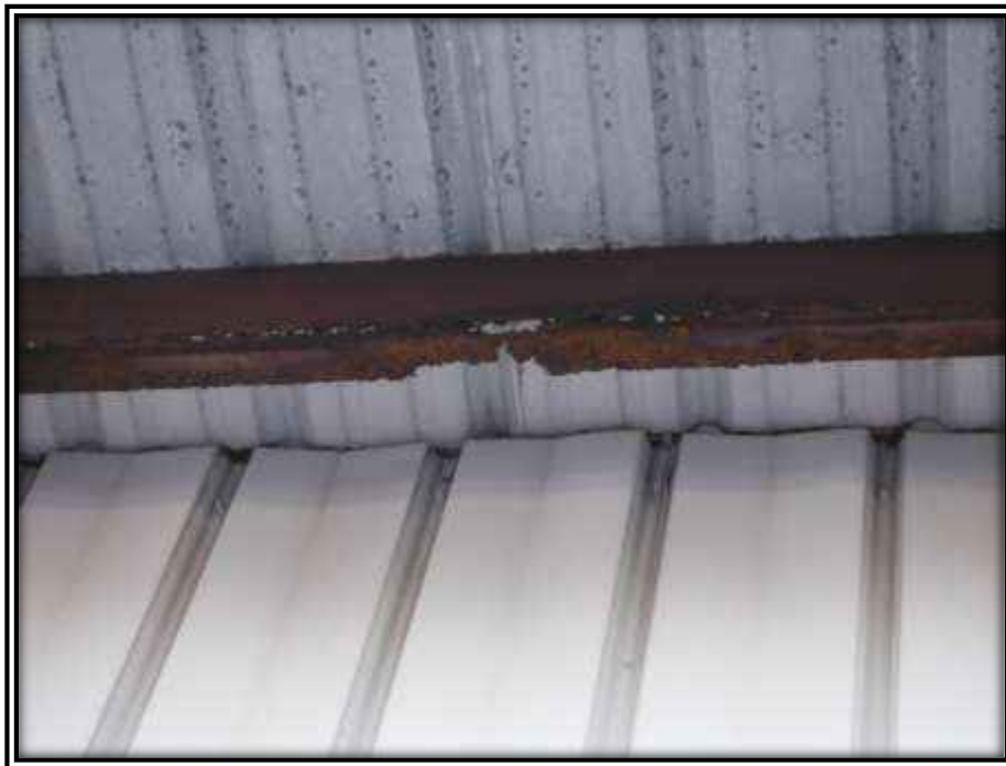
Photo E: Long-term moisture intrusion can have hidden life safety concerns as seen in the photo above where the steel purlin has no structural integrity.
