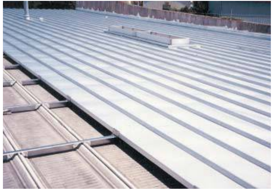
New panels being installed over Roof Huggers on an old roof (above).
