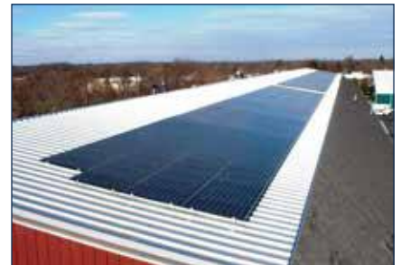
Solar panels on a standing-seam metal roof
