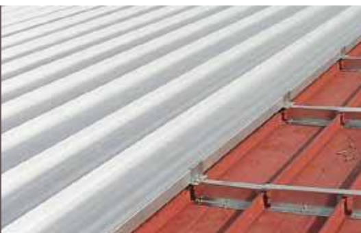
Vertical rib standing seam roof being installed over an old vertical rib standing seam roof.
