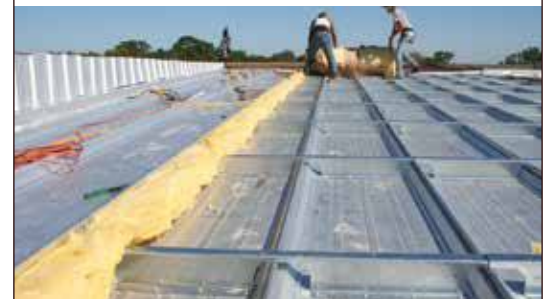
A trapezoidal standing seam roof being installed with optional insulation over an old trapezoidal standing seam roof.
