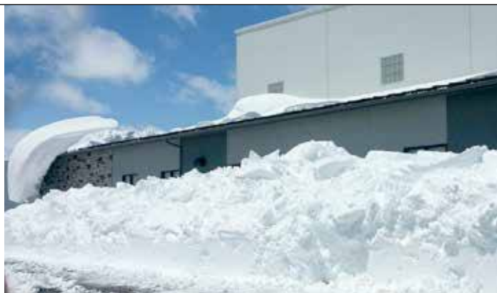
The shape and pitch of the roof and any steps in the roof will affect how snow accumulates on the building and the loads on the roof panels.
