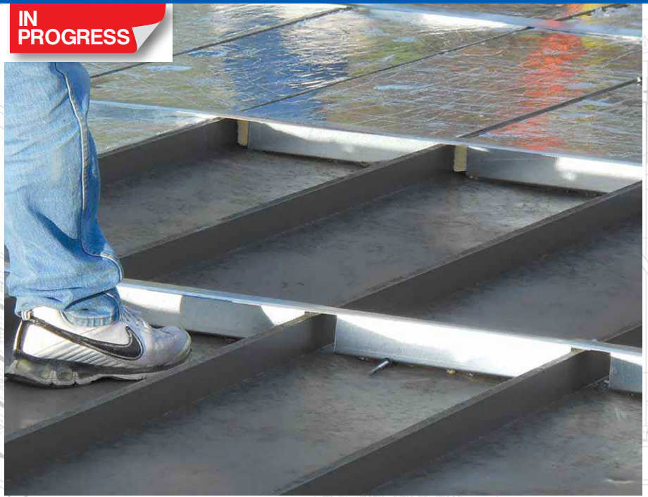
Sub-purlins have been installed as part of the metal-over-metal retrofit, and rigid insulation board is placed over the existing roof to meet current code requirements.
